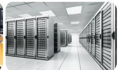
• Data Center & Server Room
