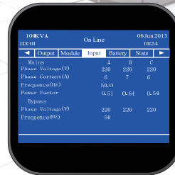
UPS Cabinet HMI Panel
